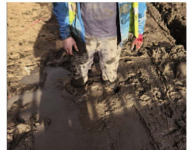
Serious flooding issues in housebuilder garden
