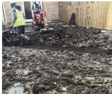
Serious flooding issues in housebuilder garden
