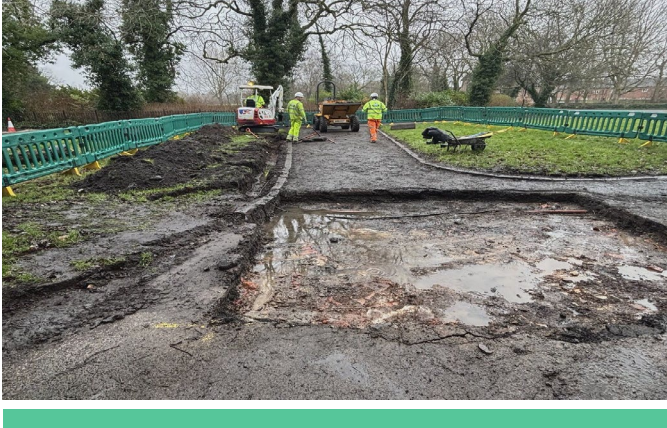
Before / during works: waterlogged conditions
