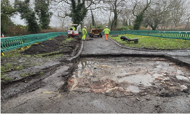
Before / during works: waterlogged conditions
